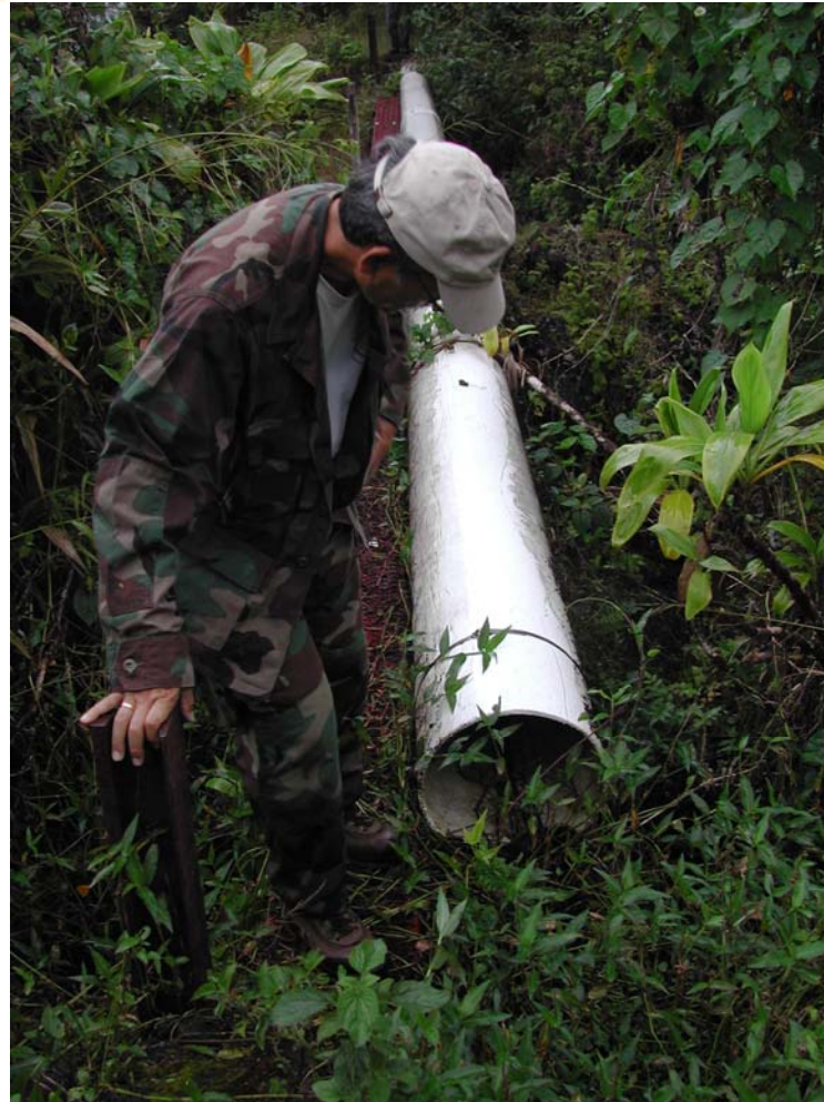
Main Kikokiko 6-in intake pipe - severed and no longer operational
