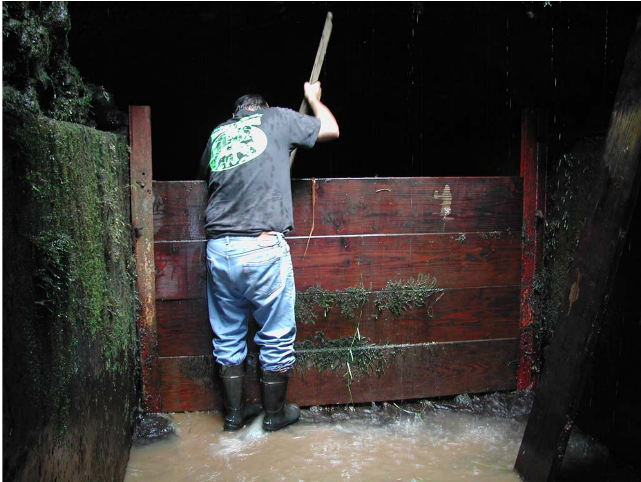
EMI staff sealed leak at K-23, #11 intake with mud and vegetation
