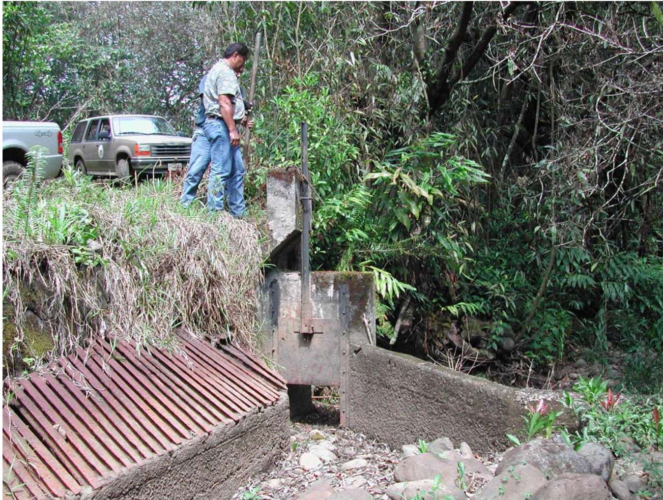
Sluce gate opening is 2-ft(W) x 1.37-ft(H)
